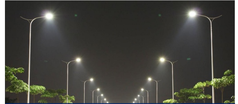
Lighting and Telecommunications
